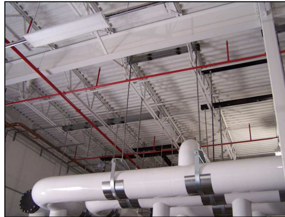
FGCU South Village Central Energy Plant Fort Myers, FL
